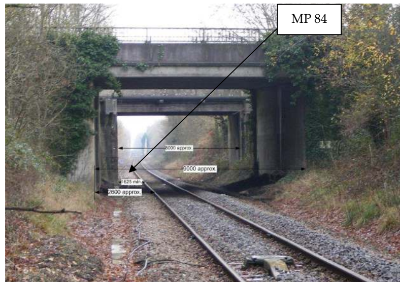
Figure 7 - Overbridge TTF-E18 2B (Main Road, 83m72Ch) with approx. clearances looking south-east towards Jacob's Gutter Lane. Station location behind both bridges (to left only for Option 1).
